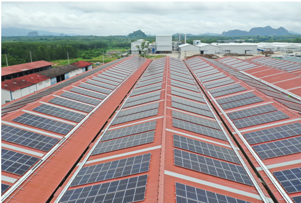
Vanachai Panel Industries Company Limited (Subsidiary), Surat Thani Factory - Electricity Generation from Solar Rooftop Project
