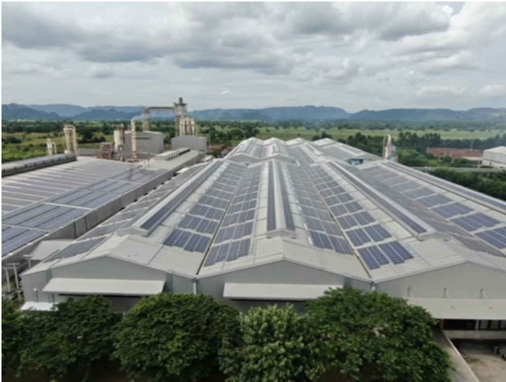
Vanachai Group Public Company Limited, Saraburi Factory - Electricity Generation from Solar Rooftop Project
